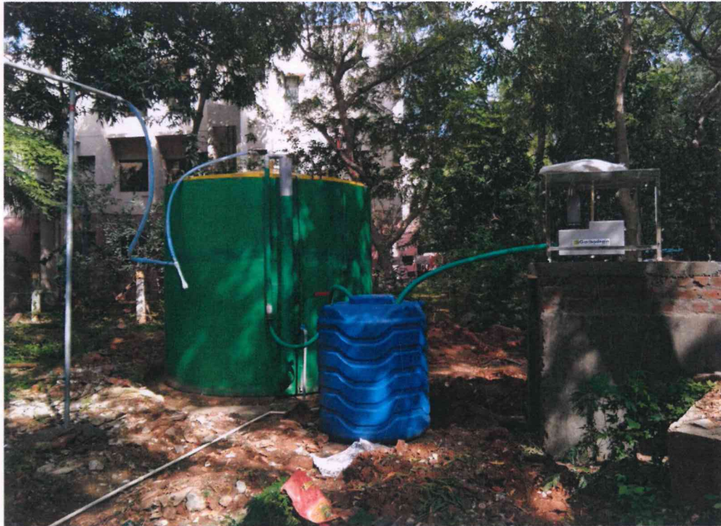
Biogas Plant in Hostel
