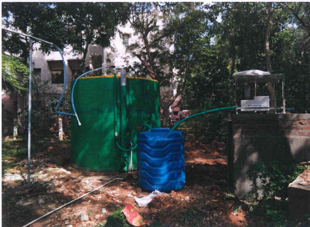
Biogas Plant in Hostel
