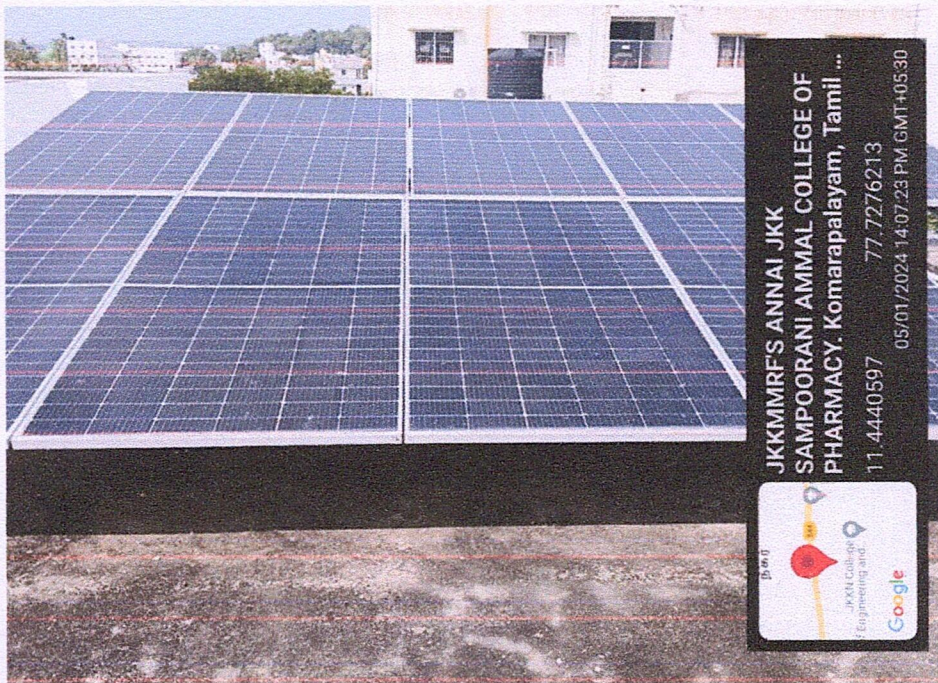
Solar Rooftop Plant
