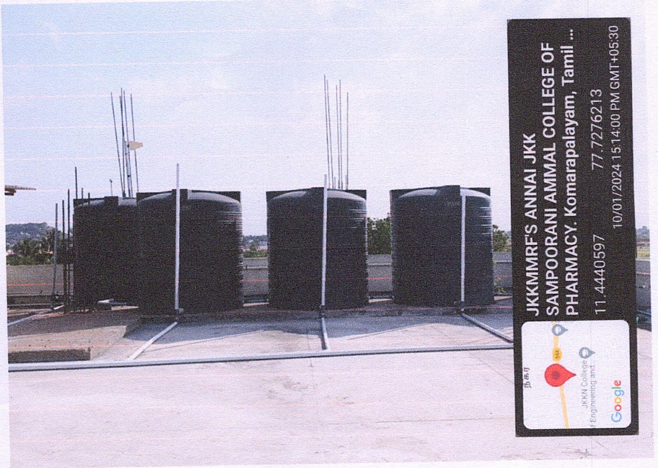
Water Storage tanks
